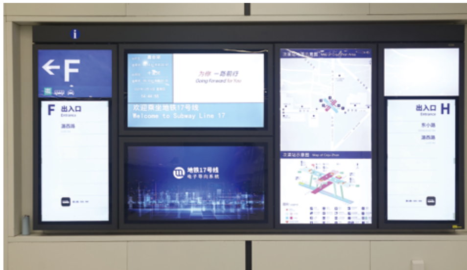
LCD screen on the wall of the BJL17 station concourse
