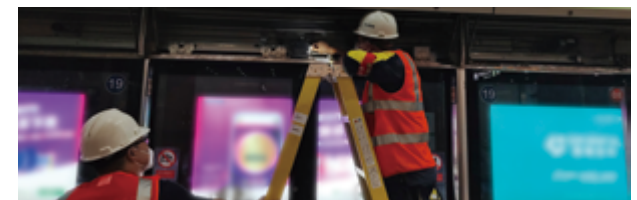
Maintenance of electromagnetic lock wire series
