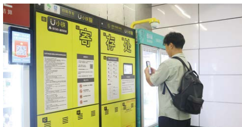
Deployment of Smart Lockers at Stations
