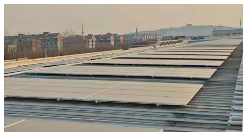
Longbeicun Depot Distributed Photovoltaic Pilot Project
